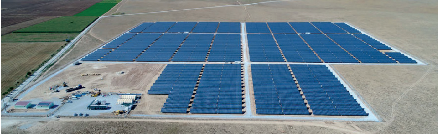
8,6 MW Konya 1 Energy Plant
