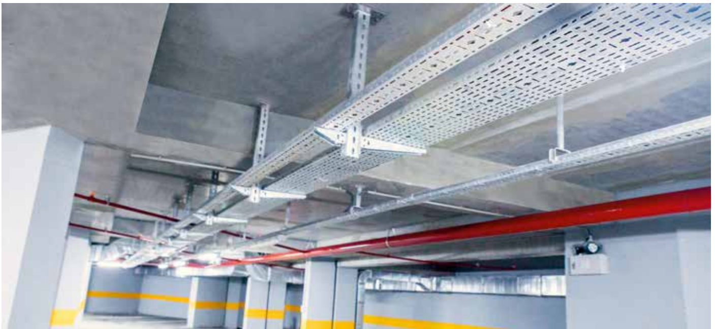
Cable tray application
