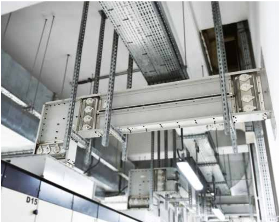
LV busbar application
